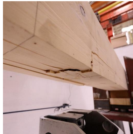
(c) Underside of specimen after failure
