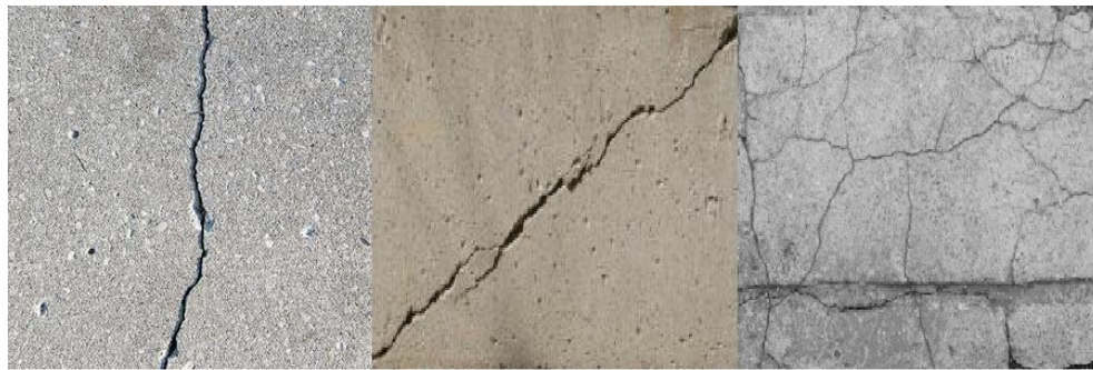
(a) Vertical/Horizontal Crack
